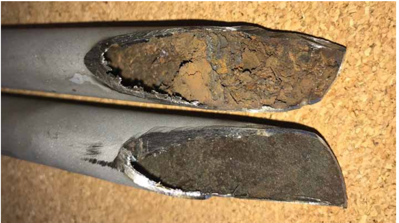
Rust was clearly present in all of the seven tubes replaced by Loree Air.
